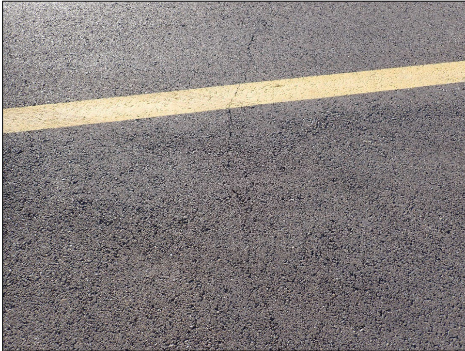
TW-11-01: L&T Cracking
