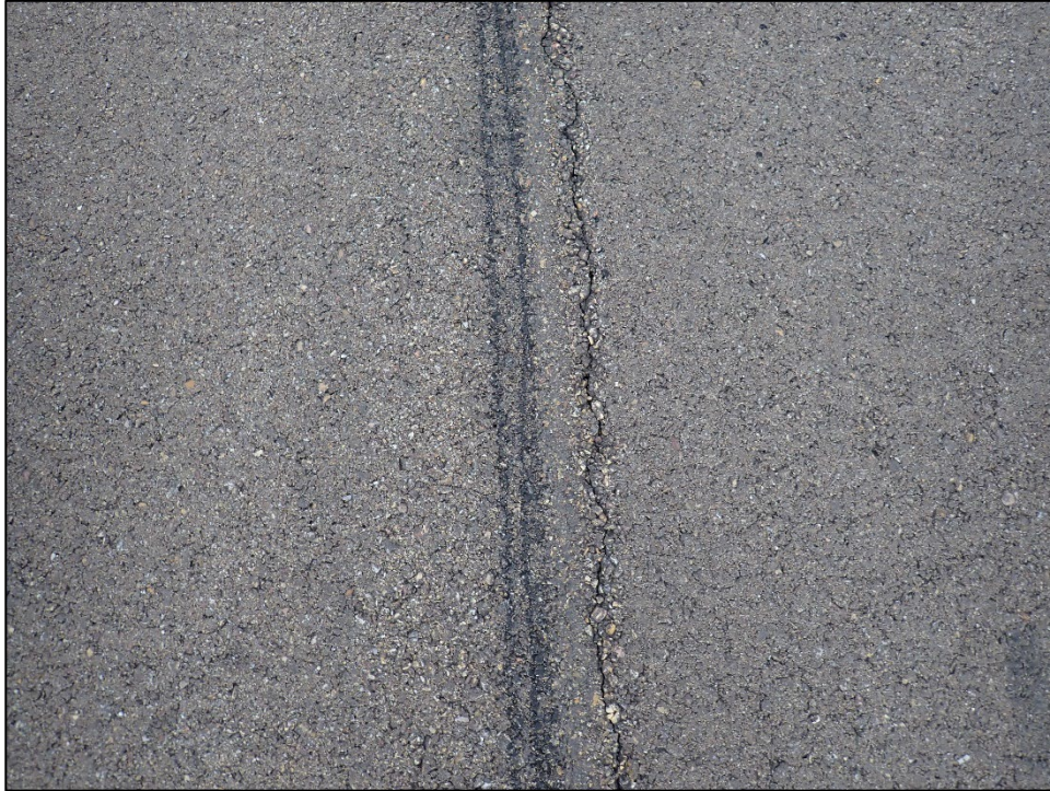
RW11-11-50: L&T Cracking
