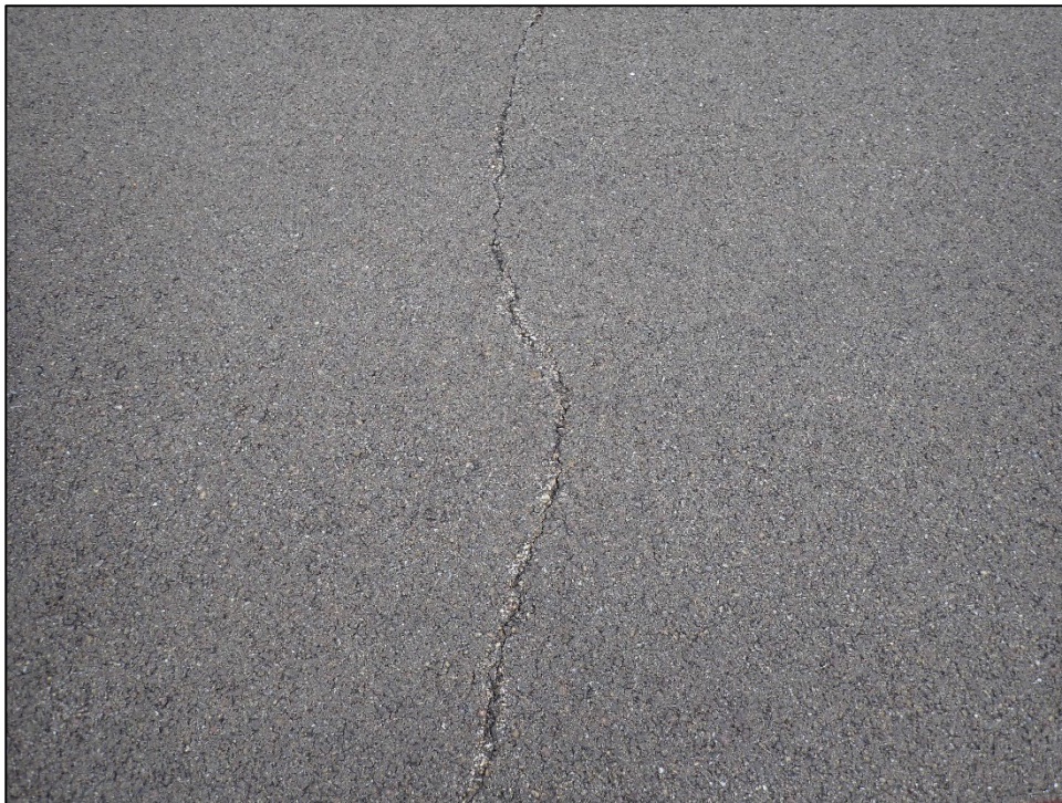
RW11-12-04: L&T Cracking
